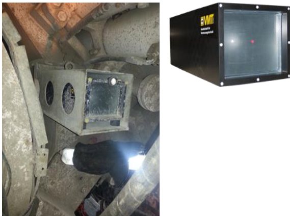
Figure 14: Automatic Laser Target Unit (ALTU)
